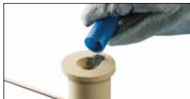
Fig. 14 Pour the starting material onto the Cadweld One Shot cover. NOTE: Welding material is an exothermic mixture and reacts to produce hot molten material with temperatures in excess of 2500 degrees Fahrenheit (1400 degrees Celsius) and a localized release of smoke. Avoid direct eye contact with "flash" of light from ignition of starting material. Avoid inhalation of smoke/fumes.
