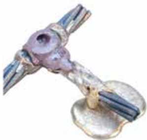
Reject. A worn or incorrect mold was used, allowing leakage around conductor. The fill in this connection is insufficient to allow it as acceptable. Replacement of mold is required prior to making next connection.
